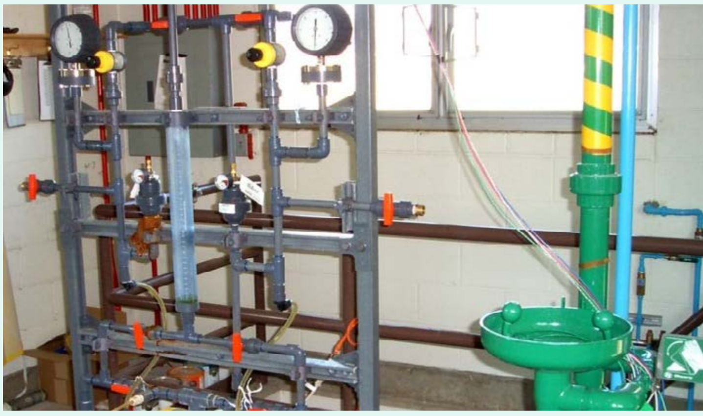
Chemical treatment for Battle Ground force main (2004)
