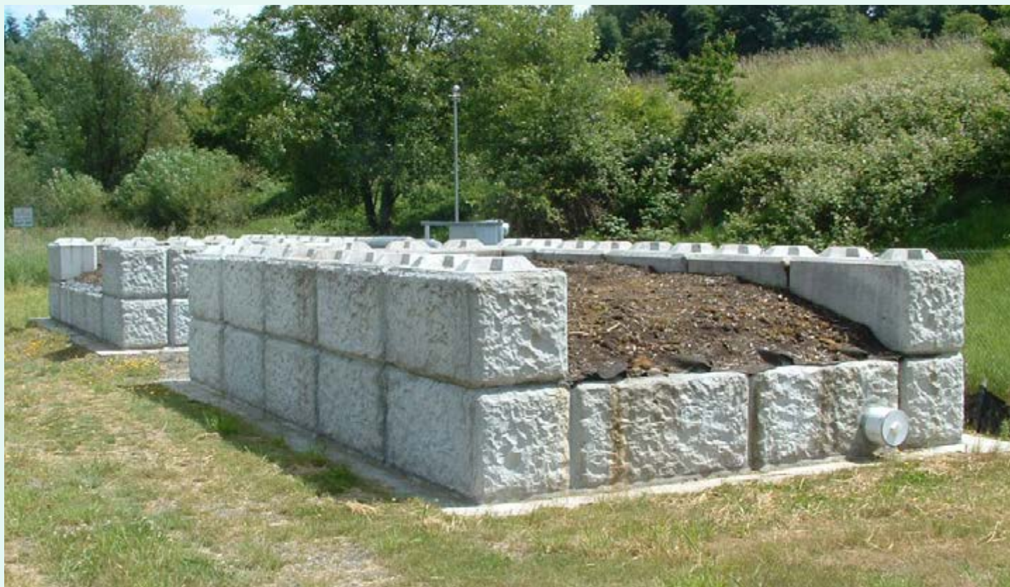
Biofilter for St Johns Interceptor (2004)
