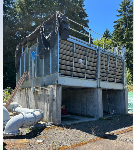
Effluent cooling tower example: Wilsonville, OR WWTP
