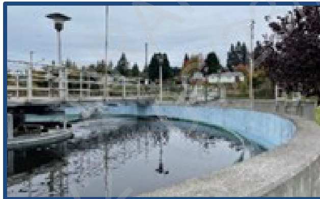
RTP Secondary Clarifier
