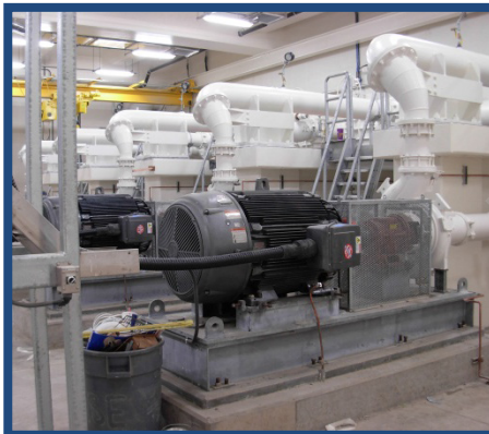
Existing Pump Assembly
