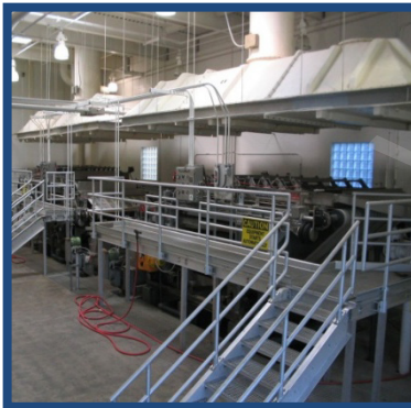
Existing SCTP Belt Filter Press
