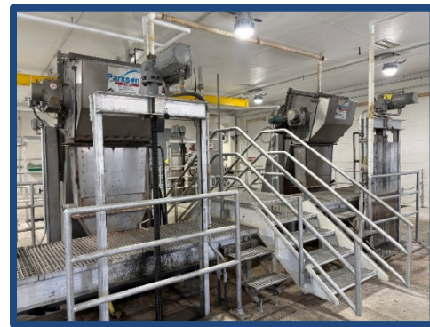
Existing Influent Screens – Back Side
