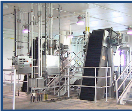
Existing Influent Screen
