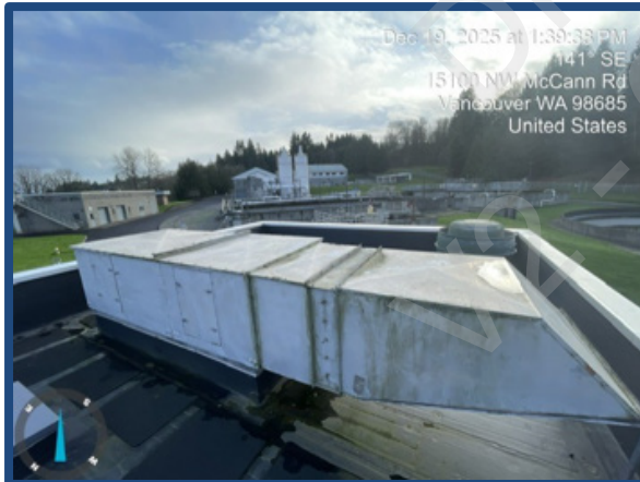
SCTP Building 47 Rooftop Air Supply Unit
