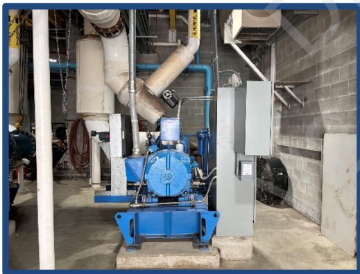
Existing Aeration Basin Blower #5
