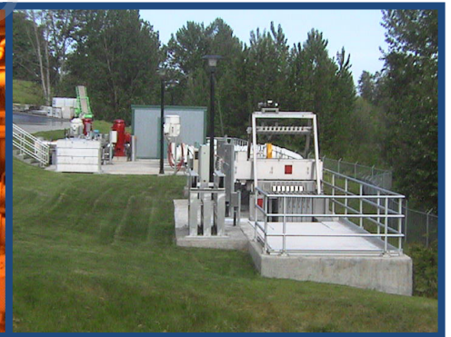
Existing UV Disinfection
