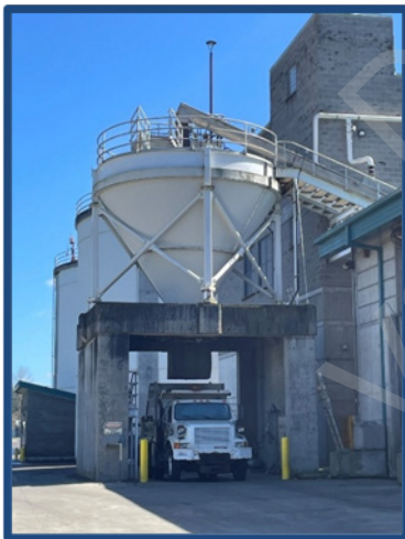
Existing Solids Hopper - Overall
