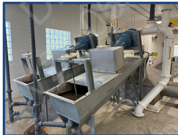
Existing Grit Classifier and Conveyor System
