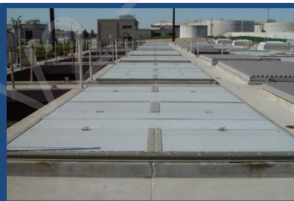
Primary Clarifier Covers
