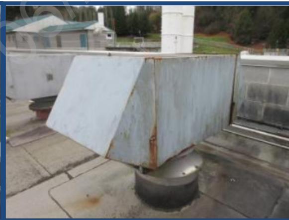
SCTP Corroded Supply Fan
