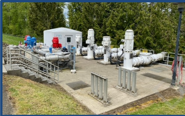
Existing Effluent Pump Station
