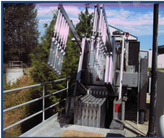
Existing UV System
