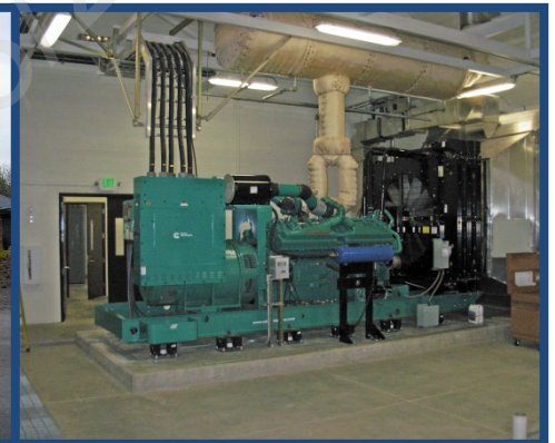
Existing Engine Generator
