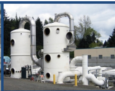
Bio Trickling Filter Tower
