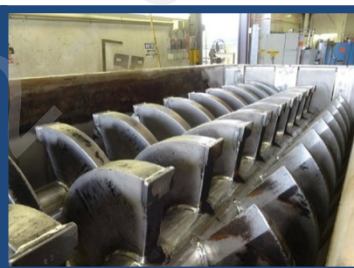
Paddle Dryer - Interior View
