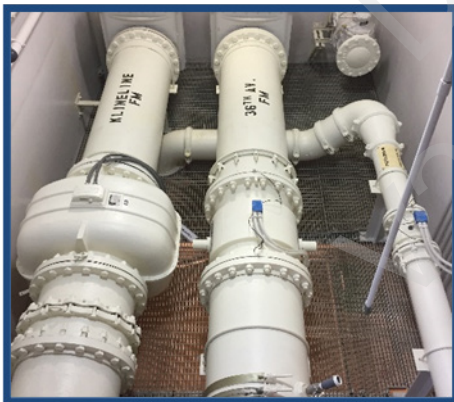
Existing Influent Flow Sensors
