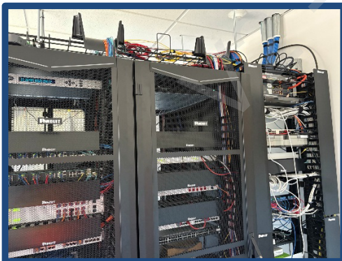
Existing Operational Technology Server Room
