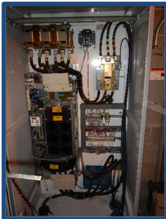
Example VFD Panel Interior
