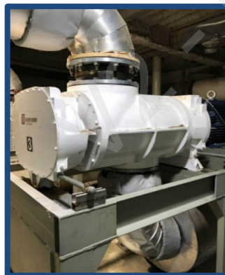
Existing Positive Displacement Blower
