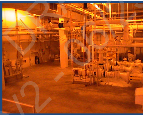
Existing RAS/WAS Pump Station
