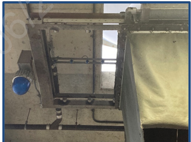
Existing Solids Hopper – Gate Position Proximity Switches
