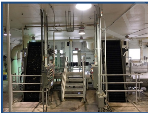
Existing Influent Screens – Front Side
