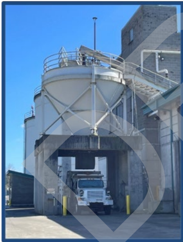
Existing Solids Hopper - Overall
