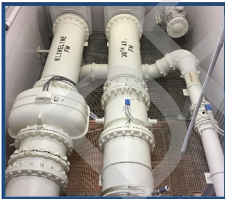
Existing Influent Flow Sensors
