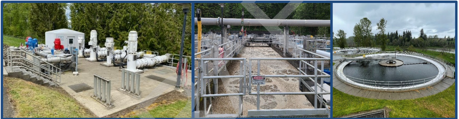
Existing Effluent Pump Station
