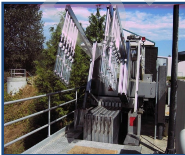
Existing UV System
