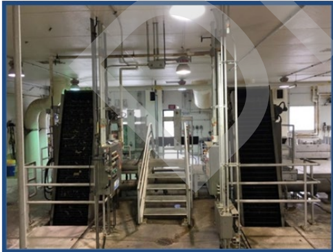
Existing Influent Screens – Front Side
