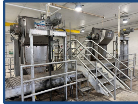
Existing Influent Screens – Back Side
