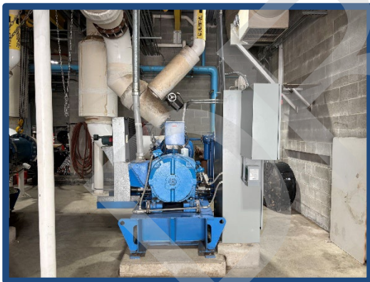
Existing Aeration Basin Blower #5
