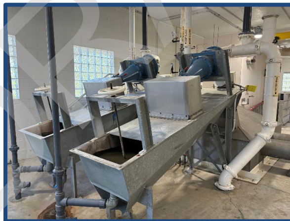
Existing Grit Classifier and Conveyor System
