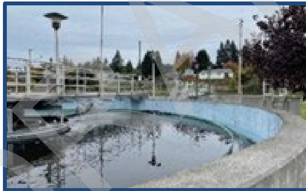
RTP Secondary Clarifier
