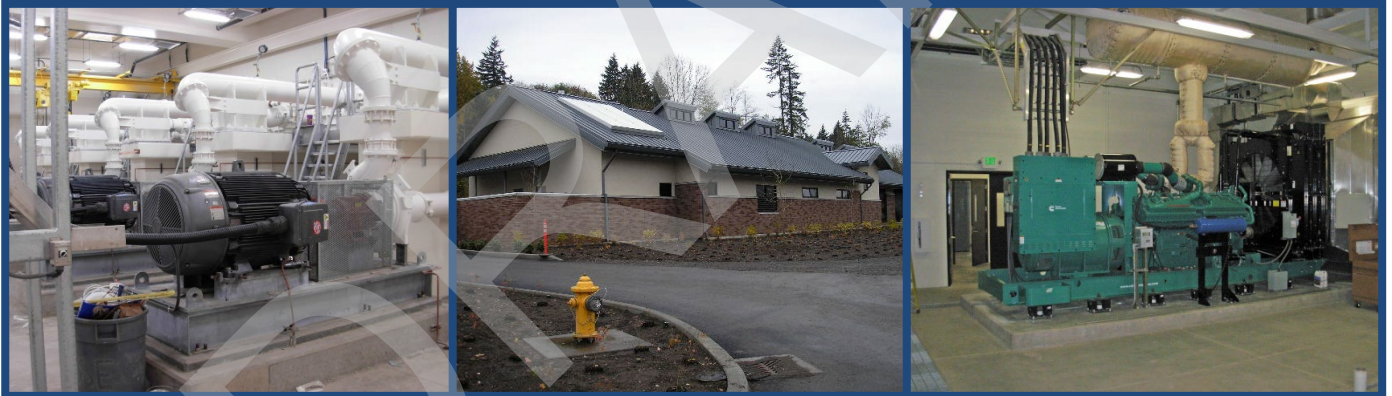
Existing Pump Assembly
