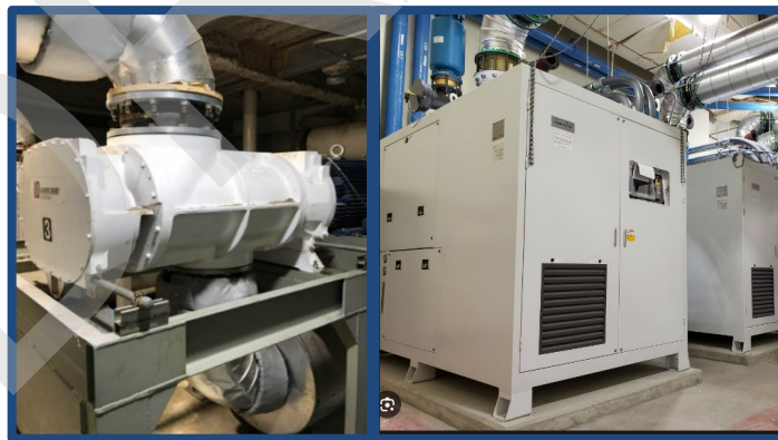
Existing Positive Displacement Blower
