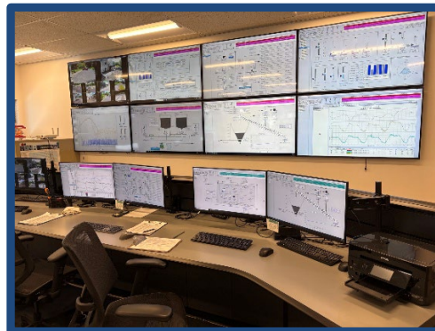
SCADA Control Room
