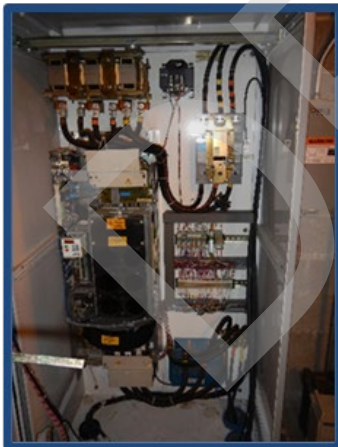
Example VFD Panel Interior
