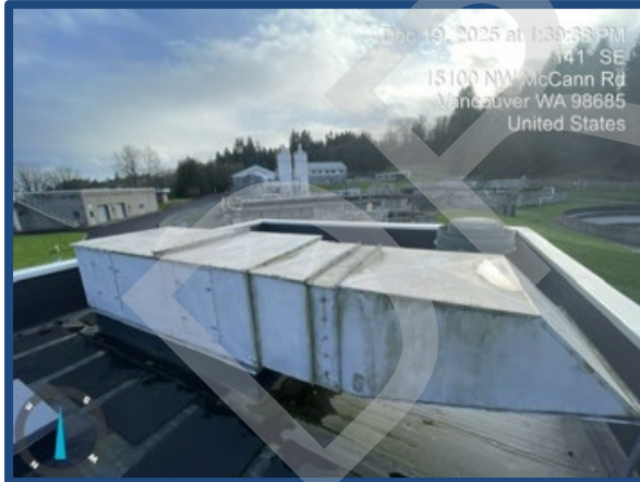
SCTP Building 47 Rooftop Air Supply Unit
