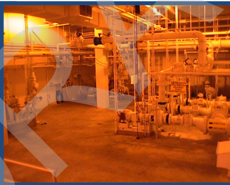
Existing RAS/WAS Pump Station
