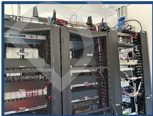
Existing Operational Technology Server Room
