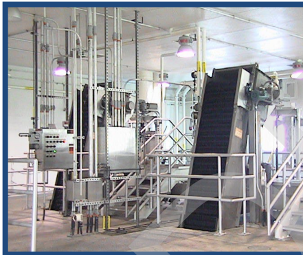
Existing Influent Screen
