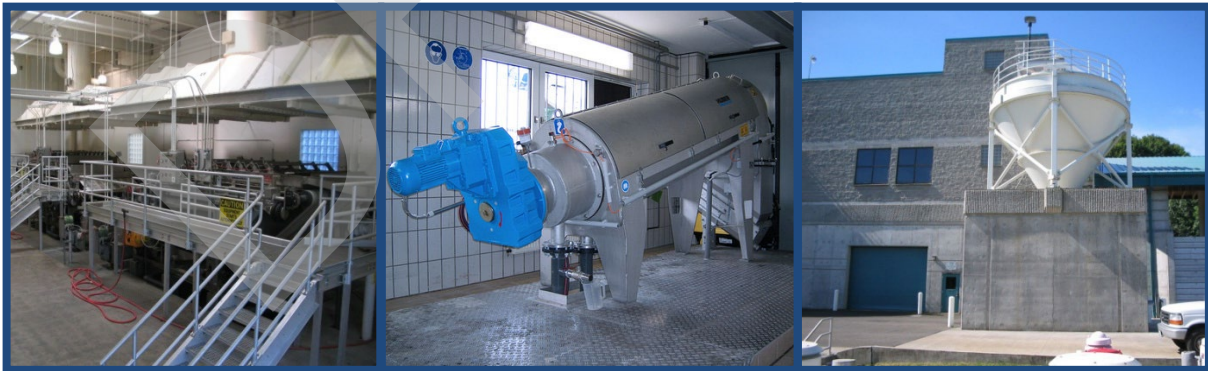
Existing SCTP Belt Filter Press
