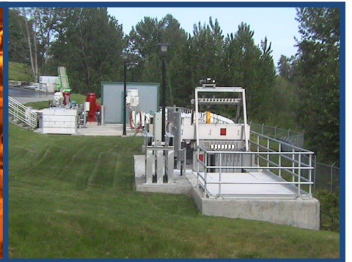
Existing UV Disinfection
