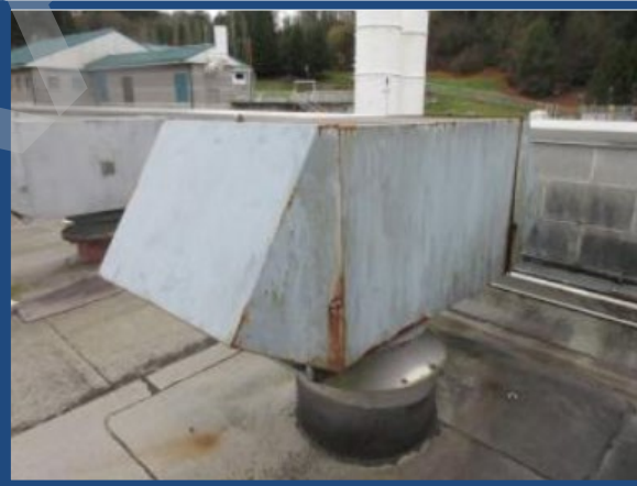
SCTP Corroded Supply Fan
