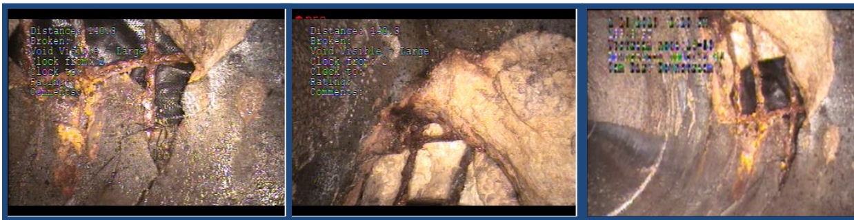
Signs of Failure of the Interceptor
