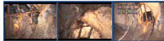
Signs of Failure of the Interceptor
