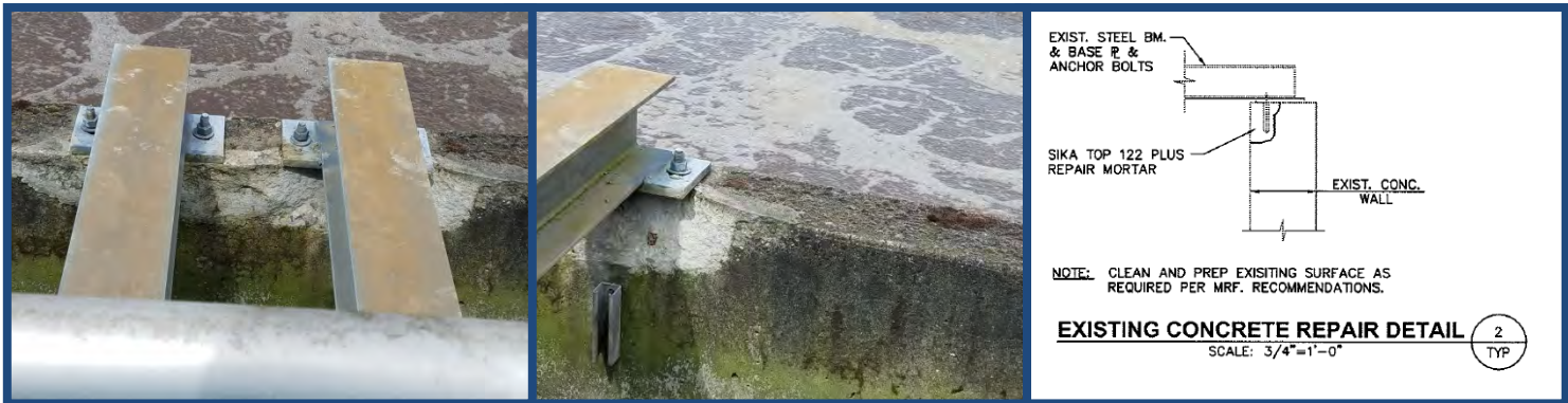
Failed Concrete at Aeration Basin Mixer Support
