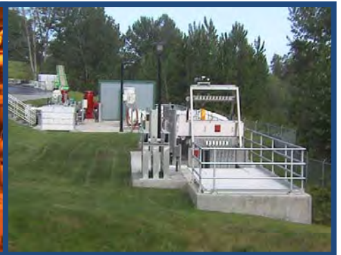
Existing UV Disinfection
