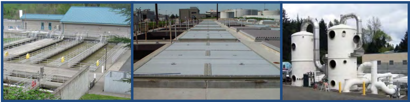
Existing Primary Clarifiers
