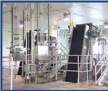
Existing Influent Screen
