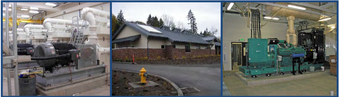
Existing Pump Assembly
