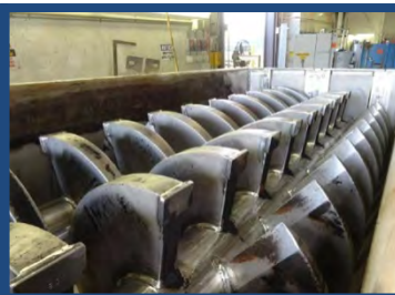
Paddle Dryer - Interior View
