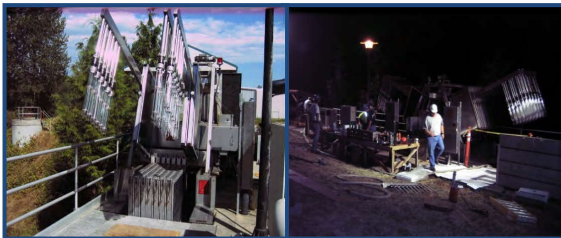
Existing UV System
