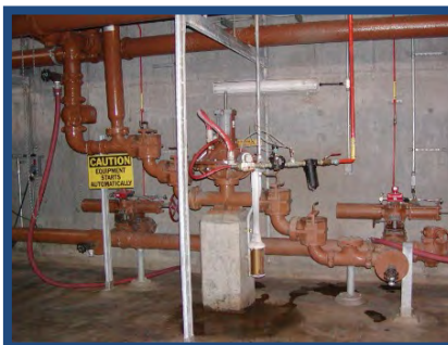
Existing Diaphragm Style Pump
