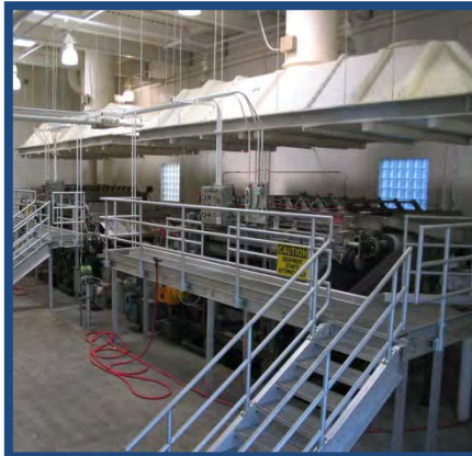
Existing Sctp Belt Filter Press
