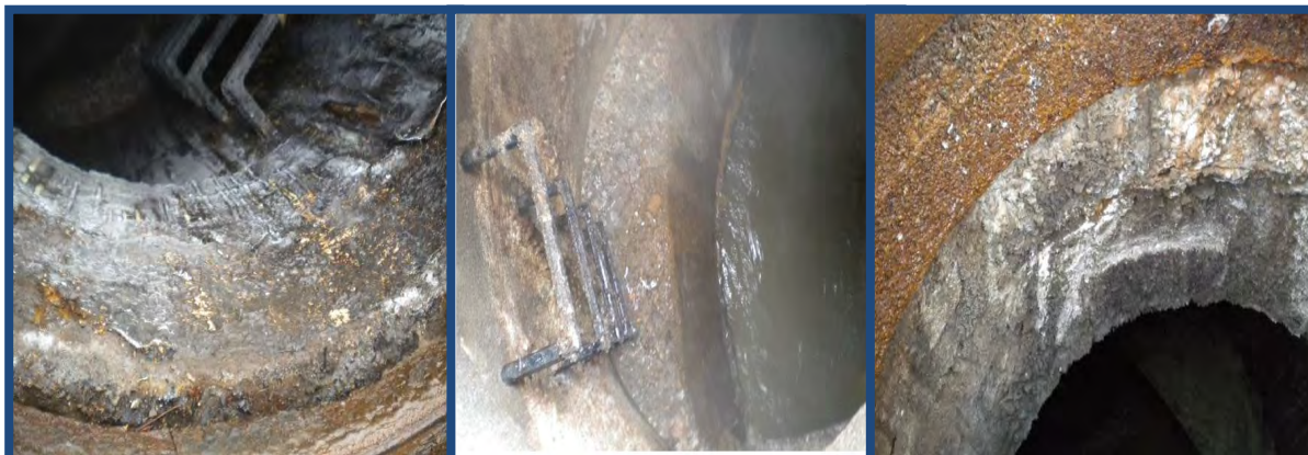
Corrosion Around Manhole Rim
