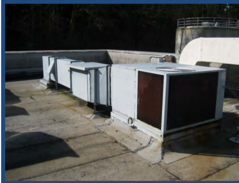
Aged HVAC Unit at Facility 37
