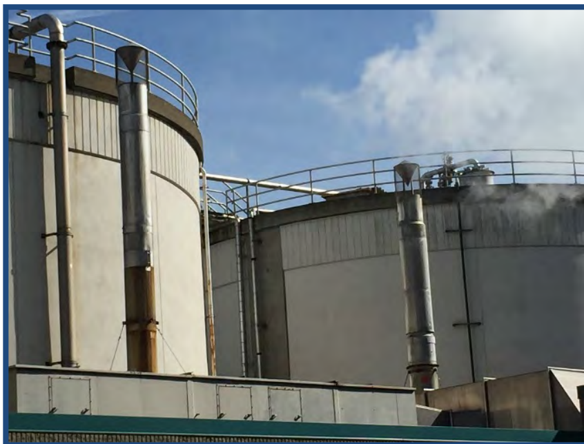
Existing Boiler Stacks
