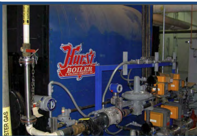
Boiler 1 with Gas Train
