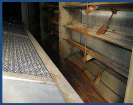
Aged HVAC Unit at Facility 70
