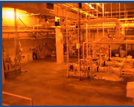
Existing RAS/WAS Pump Station
