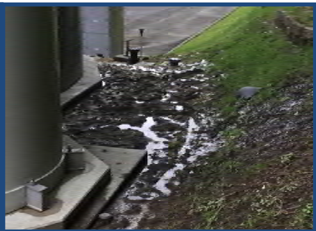
Saturated Ground At Foundation
