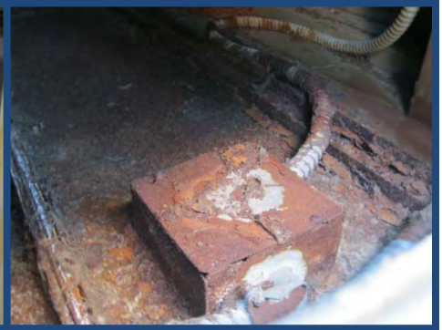
Aged HVAC Unit at Facility 72
